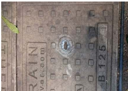
Condition of the socket type keyhole lifting arrangement of THERMODRAIN FRP manhole covers
